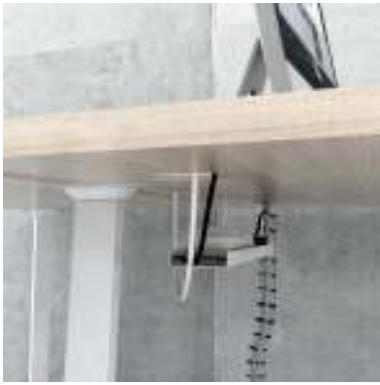
E64 HORIZONTAL CABLE TRAY
